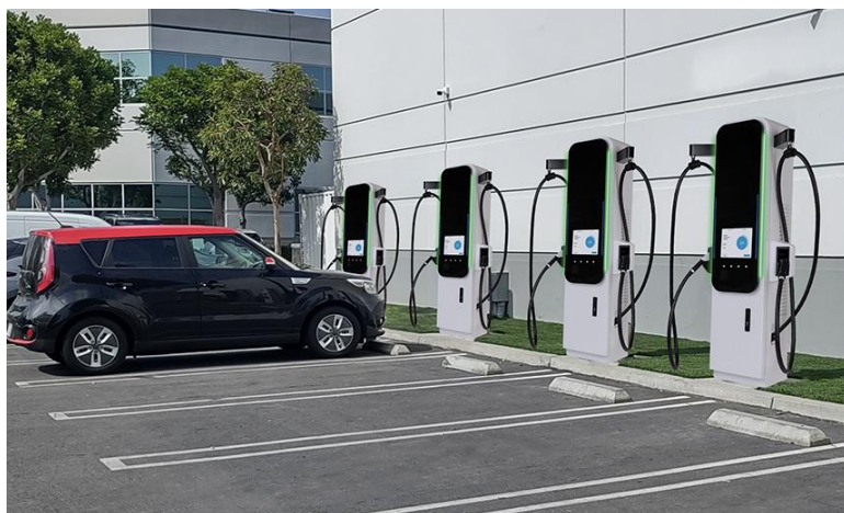
Figure 6 EV Charging station
